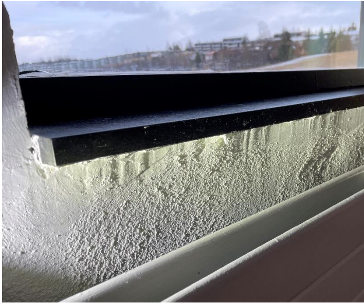
Mynd 10. Meginland, rakaummerki undir gluggum. Gluggakistur innihalda asbest.
